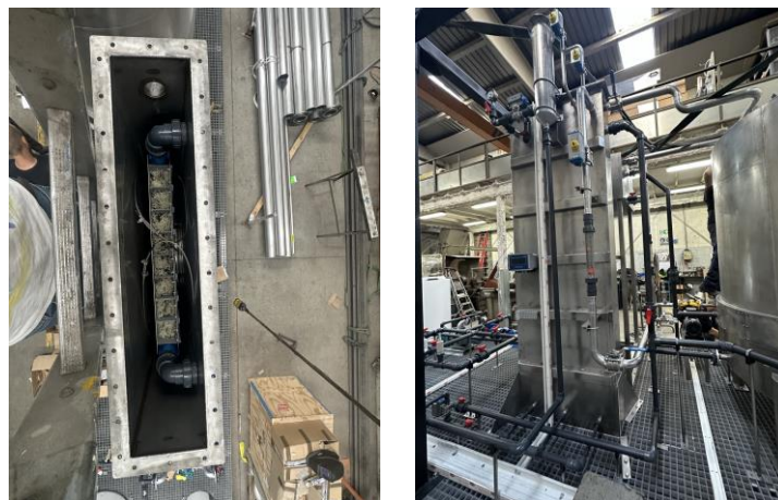
Figure 6: Commercial ultrafiltration membrane reactor (KOCH) installed at the Spanish EcoSite.
