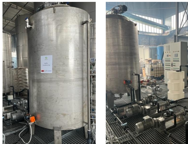
Figure 24: Greek EcoSite conditioning tank.
