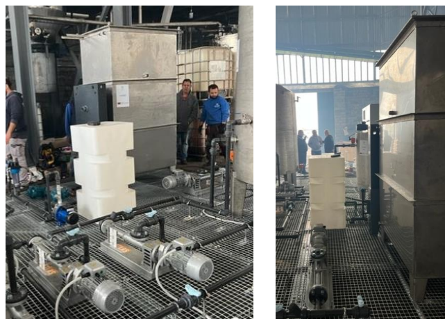
Figure 26: Membrane unit built and installed in the Greek EcoSite.
