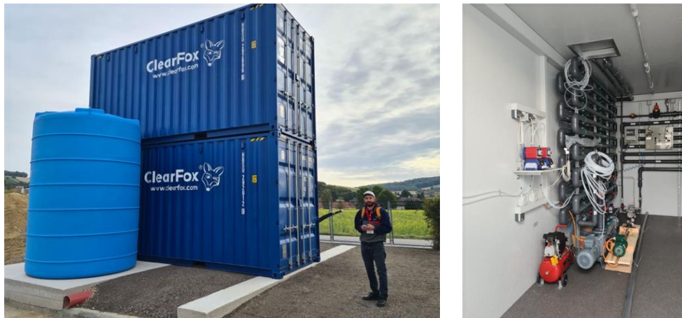
Figure 10: Flotation unit installed at the Austrian EcoSite.
