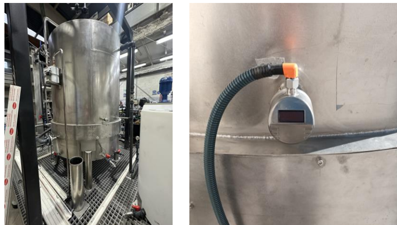
Figure 4: Anaerobic digester of the AnMBR system of the Spanish EcoSite.
