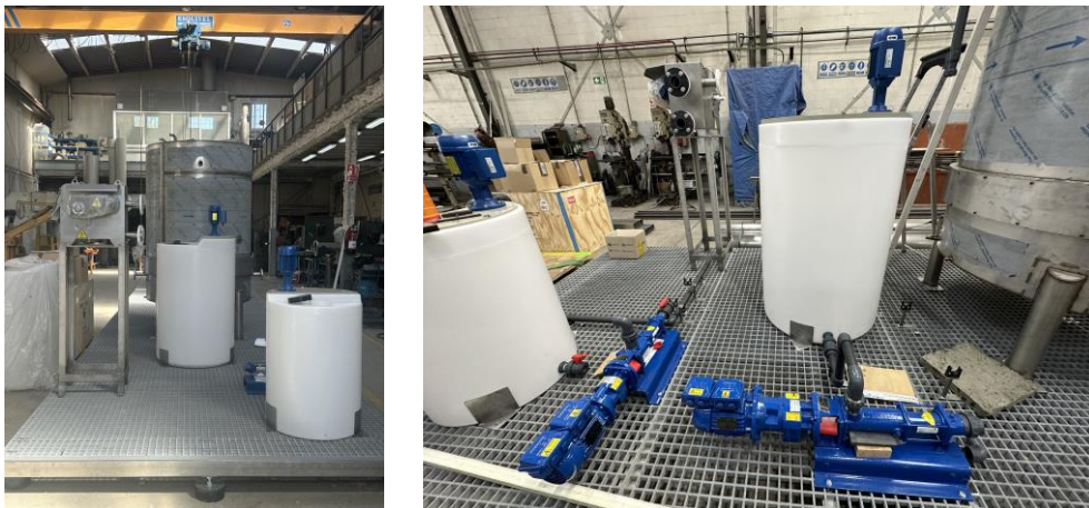
Figure 2: Rotary sieve (left) and auxiliary components installed on the GRP platform in the Spanish EcoSite (right)
