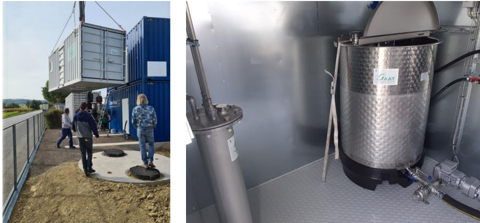
Figure 12: Container for the biogas production stage and substrate tank installed at the Austrian EcoSite.
