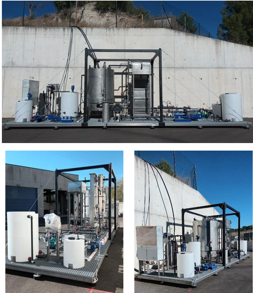
Figure 9: Pilot plant of the Spanish EcoSite integrated into its final location at the Alcoy WWTP.
