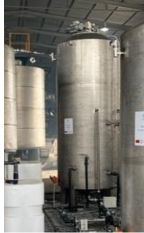
Figure 25: Anaerobic digester (CSTR2) installed in the Greek EcoSite pilot plant.
