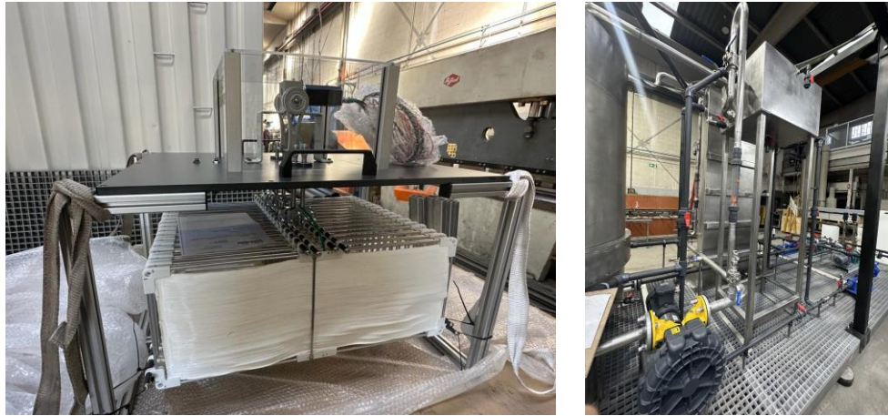
Figure 7: Membrane reactor with MMV system (KUL) installed in the Spanish Ecosite.
