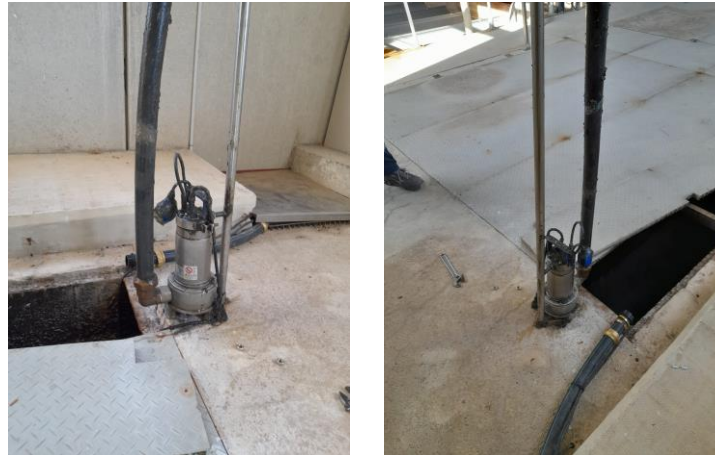
Figure 3: WW drive pump installed at the Spanish EcoSite.
