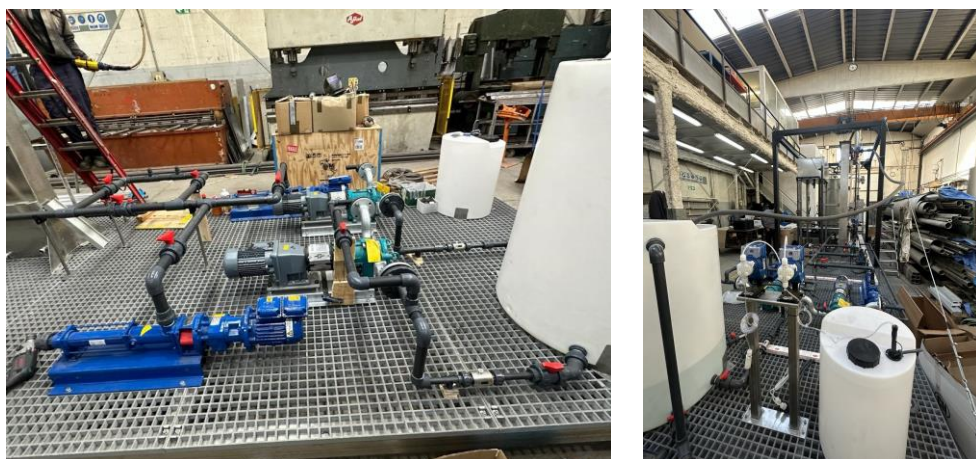
Figure 8: Auxiliary components of the membrane units of the Spanish EcoSite.
