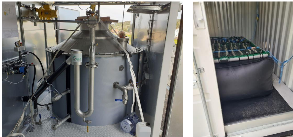
Figure 13: Biogas digester and biogas storage bag installed at the Austrian EcoSite.
