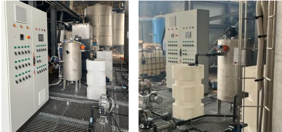
Figure 23: Dark fermentation unit (CSTR1) built and installed at the Greek EcoSite.
