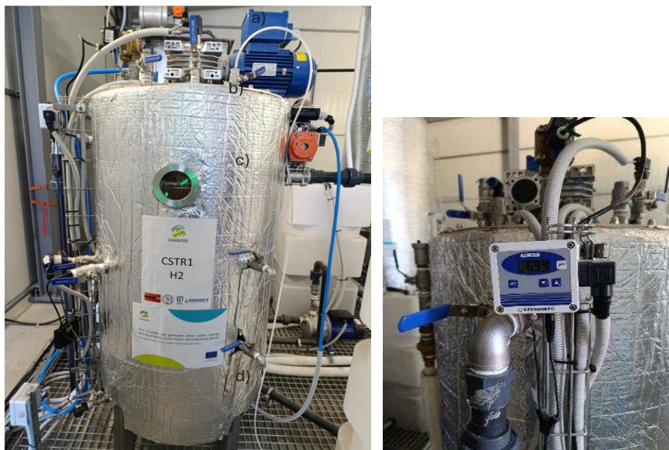
Figure 57. The 350 L pilot-scale reactor (CSTR1) installed at the Greek EcoSite
